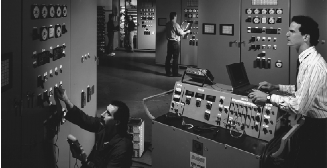
17.6 MW System Control for Cernavoda Nuclear Power Plant, Romania
