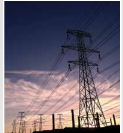
Electric utility substations Switchgear
